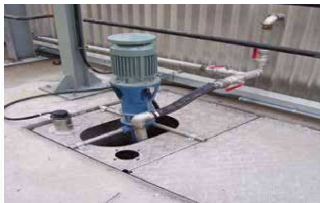
System condensate is collected and pumped back into the system for reuse.
