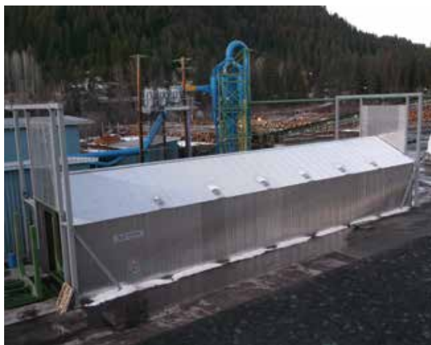
During operation both doors are opened, new logs are pushed in one end and conditioned logs are pushed out the other end.
